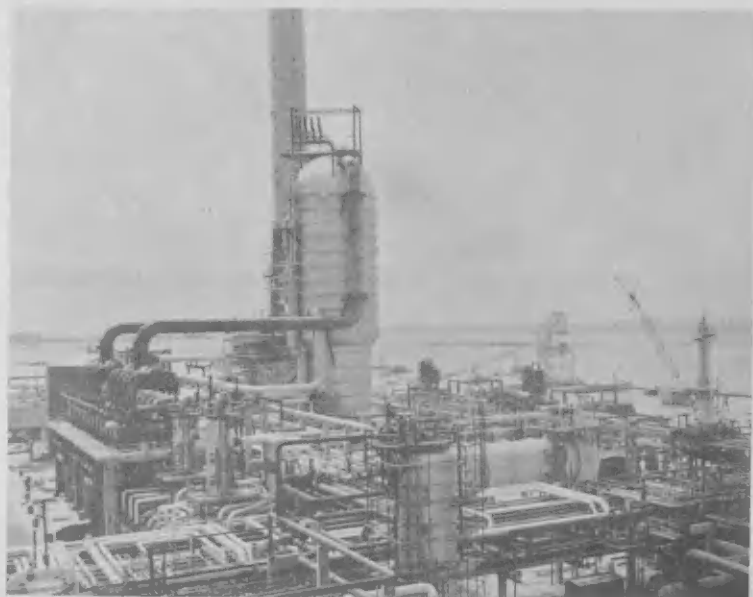
Vacuum Pipestill with HDS Process Stack.
